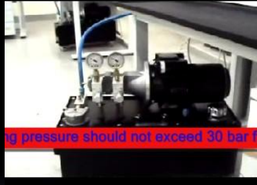
Fig. 1.13: The hydraulic power pack.
